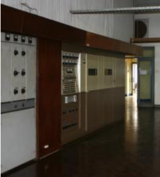
A derelict Phillips (left) stands mute alongside the new CEC at the KM6 facility. M. Guha
